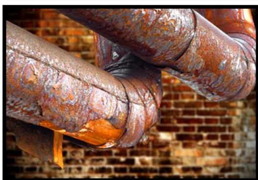
Fig 4: Corrosion in pipes
