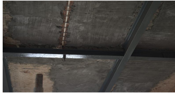
Fig.8. Injecting of cement slurry grouting (M-50 grade) & applying of two coats of zinc.
