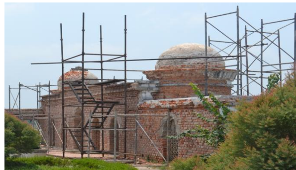
Fig.9. self-supported scaffolding double row type using steel pipes for vertical, horizontal and diagonal bracing.
