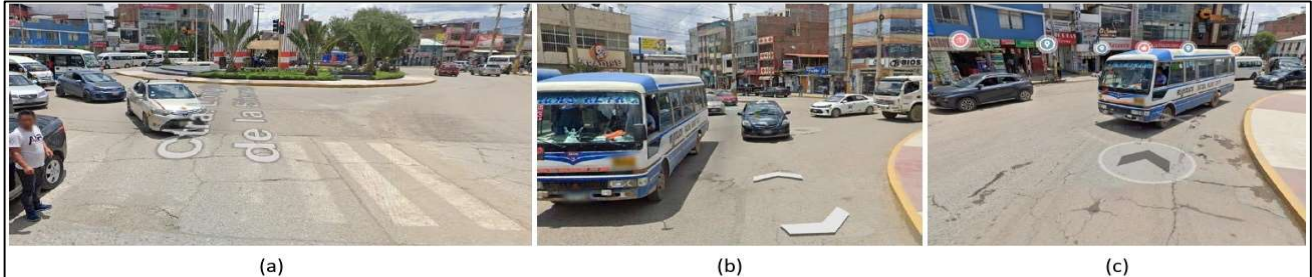
Fig. 1 Rigid pavement in poor condition
