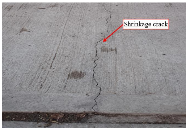
Fig. 2 Shrinkage crack in concrete, closer look [7]
