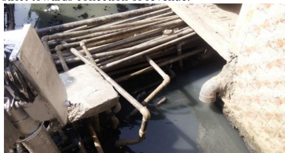
Figure 4.2 Illegal Connections in an Area
