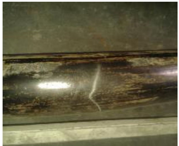
Fig.4 Failure of Columns
