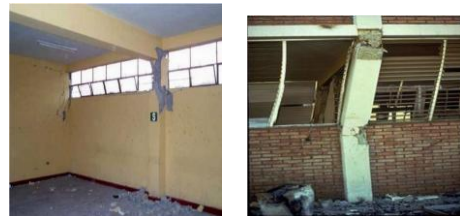
Fig. 1: Failure Pattern Due to Captive Column Effect
