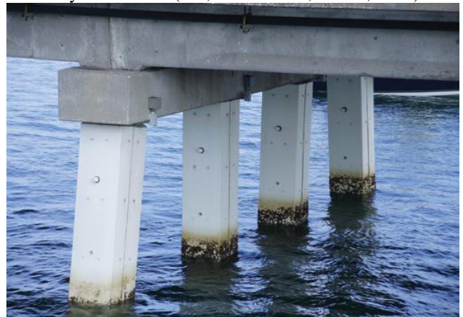
Fig. 3 An RC structure exposed to chlorides (Legault 2011)
