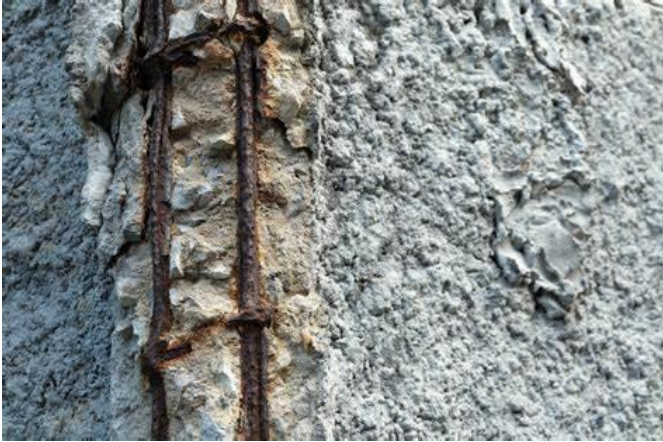
Fig. 4 Chlorides-induced corrosion (Graham 2017)
