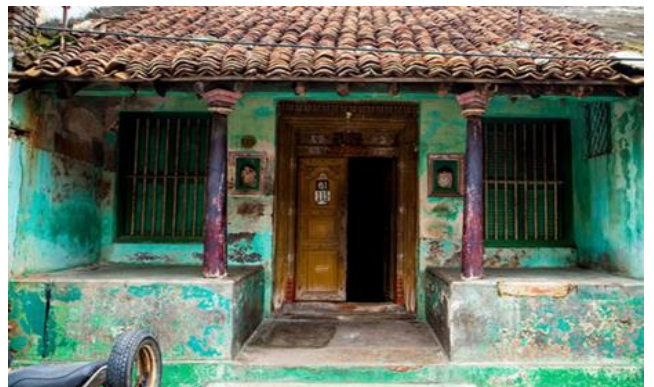
Fig. 13 Doors and windows of building facade – traditional Agraharam house at Nagercoil district
