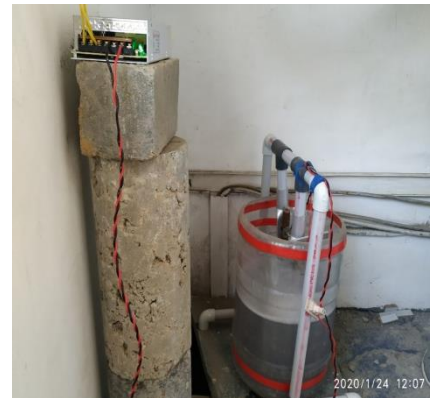
Fig. 1 Water treatment using electrocoagulation
