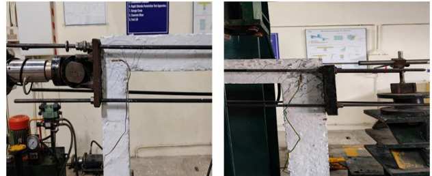
Fig. 13 Crack pattern of RC frame without damper
