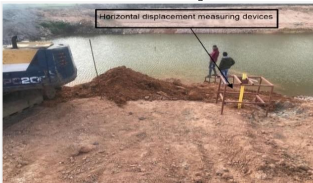
Fig. 7 The position of the inclinometer used for horizontal displacement monitoring
