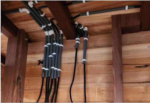
Fig. 9 Electrical installation on the pinisi tourist ship (not marine standard)
