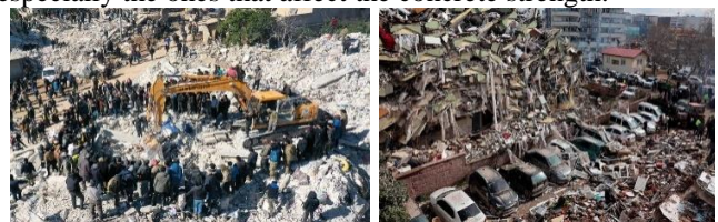
Fig. 1 Damage observed in reinforced concrete buildings during the Kahramanmaraş earthquake sequence, Turkey (2023). (1a) Collapsed building in the city of Harim, Syria, near the border with Turkey—(1b) Debris from collapsed buildings in Kahramanmaraş, near the earthquake epicenter
