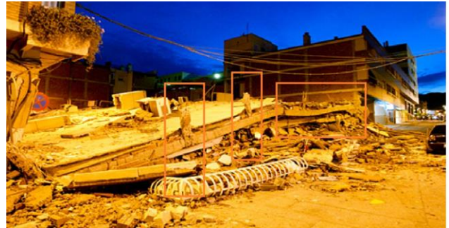
Fig. 3 Slab-column connection damage and observed in waffle slab buildings during the 2011 Lorca earthquake (Spain)
