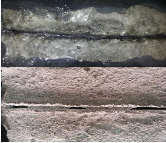
Fig. 17 Showing crack healing
