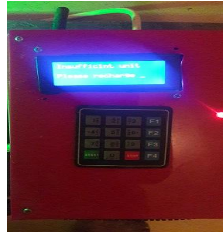
Figure 4.2: Insufficient Unit Notification on the Meter’s LCD
