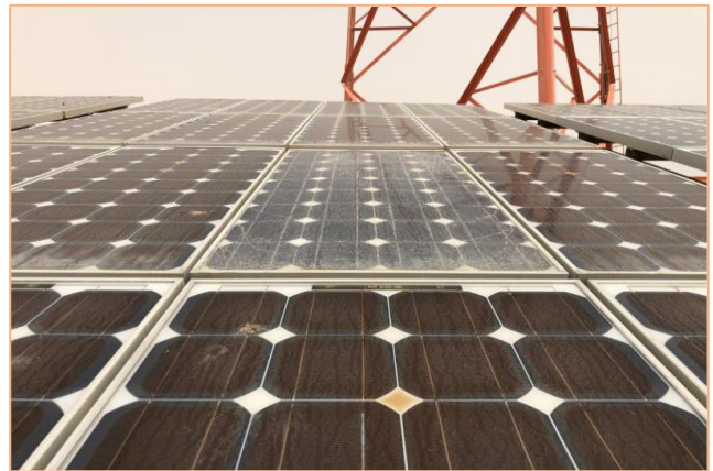
Fig. 3 Soiling and discoloration on the outside layer of modules
