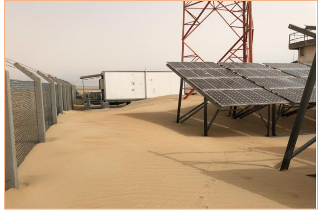
Fig. 2 Sand accumulation in one of the telecommunications repeaters
