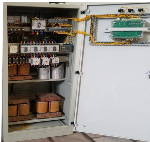
Fig. 19 The central controller embedded in the electrical control cabinet
