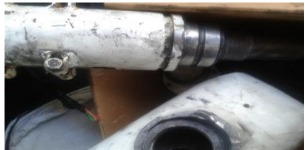
Fig. 4 Damage in the internal shaft of rotary part of wind turbine
