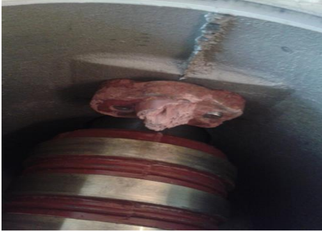
Fig. 7 Loss of contacts due to shaft damage in small wind turbine
