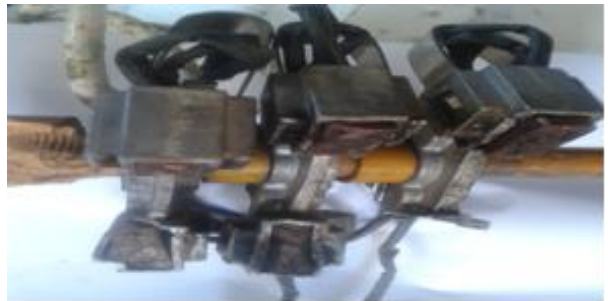
Fig. 5 Damage in the brushes and brush holders inside the rotary part
