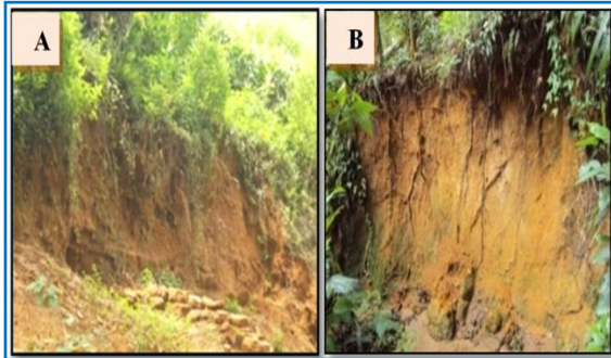
Plate 04: Cutting failures. (A) Pitakande. (B) Madakumbura, (Field survey)
