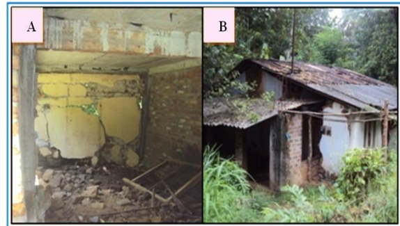
Plate 06: Houses damaged by subsidence in Mousagolla and Bodhikotuwa division (Field survey)
