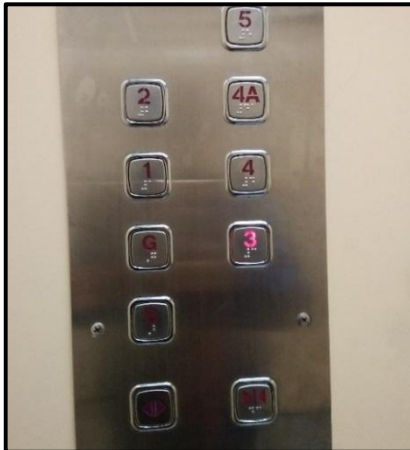
Picture 7. Braille Brace Elevator Button
