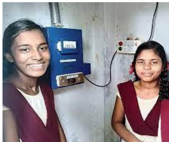
Fig. 4 School girls with a new incinerator installed in their school
