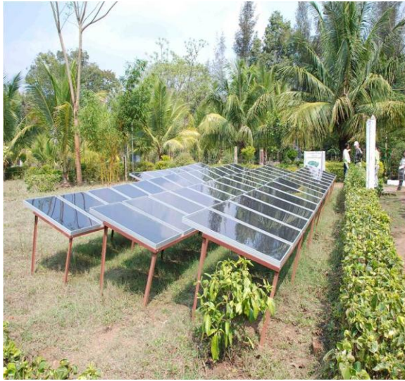
Fig.5. A solar water pump installed in Hosahalli village in Karnataka
