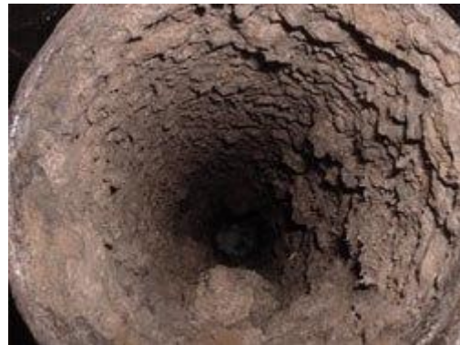
Fig. (4) - View of Biological Corrosion
