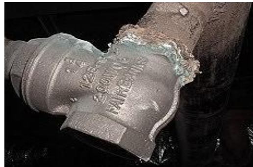
Fig (11) Galvanic Corrosion.
