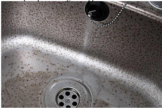
Fig (9) - An Industrial Sink Unit Where Chlorine Containing Cleaner has Caused Pitting Corrosion.
