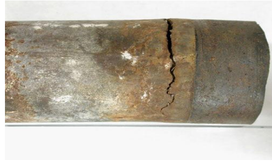
Fig (10) - Stress Corrosion
