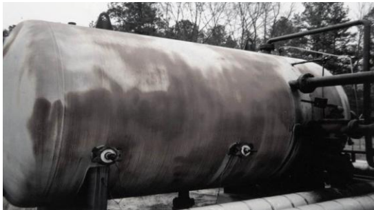
Fig (2) - Uniform corrosion
