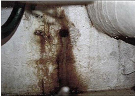
Fig (5) - Telltales of Crevice Corrosion Through Bolts.
