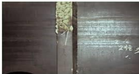
Fig (13) - Waterline Corrosion
