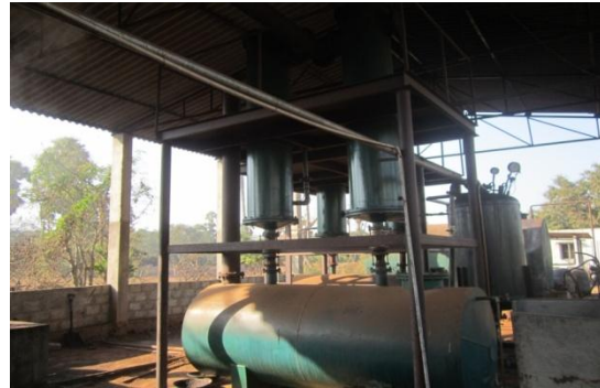
Figure 5 The Four stage Condenser set up
