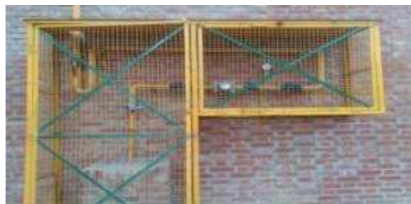
Fig 1. Mandela Hostel Mess Gas Meter
