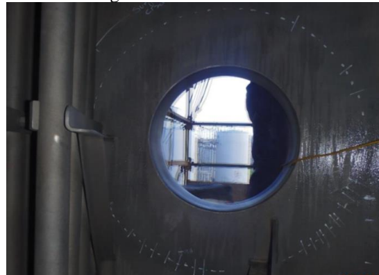
Figure 14 Cracks detected on the outer shell surface-initiated on the blind side of the shell and corresponding re-pad (photo taken from inside of vessel)
