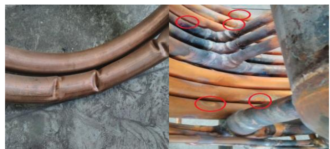
Fig. 1 HCHE wrinkled pipes
