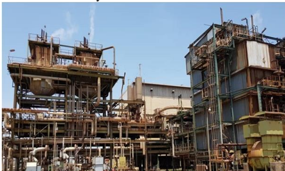
Fig. 1: KRPC steam power plant
