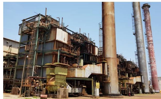
Fig. 2: KRPC steam power plant boilers
