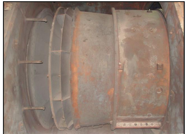
Gas Turbine exhaust / thermocouples
